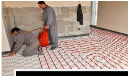
Under floor heating
